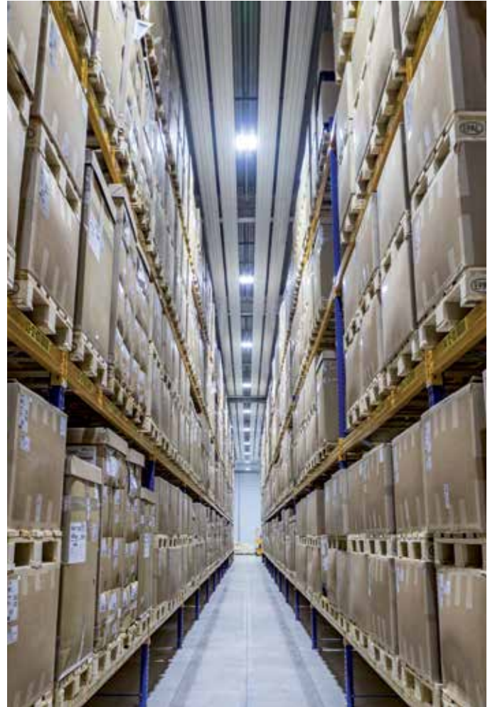
The radiant ceiling panels make even heat distribution possible, so that no heat accumulation occurs under the hall ceiling. In the event of a fire, this ensures better smoke extraction. This meant that there was no need to install an expensive and complex fire alarm system in the warehouses. Instead, only a few conventional smoke detectors were needed.
